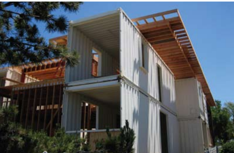
This 3,500-sq.-ft home in Redondo Beach, Calif., designed by Architect Peter DeMaria, uses eight ISBUs.
