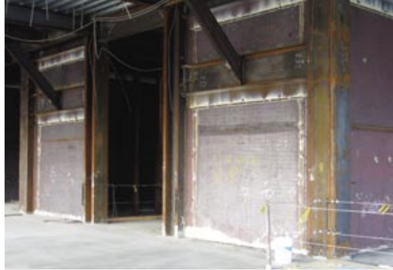
Above: In locations where the code-prescribed aspect ratio of the steel plate panel was not naturally achieved, KPFF added intermediate horizontal boundary elements (HBEs) with wide-flange steel kickers between floor levels.
