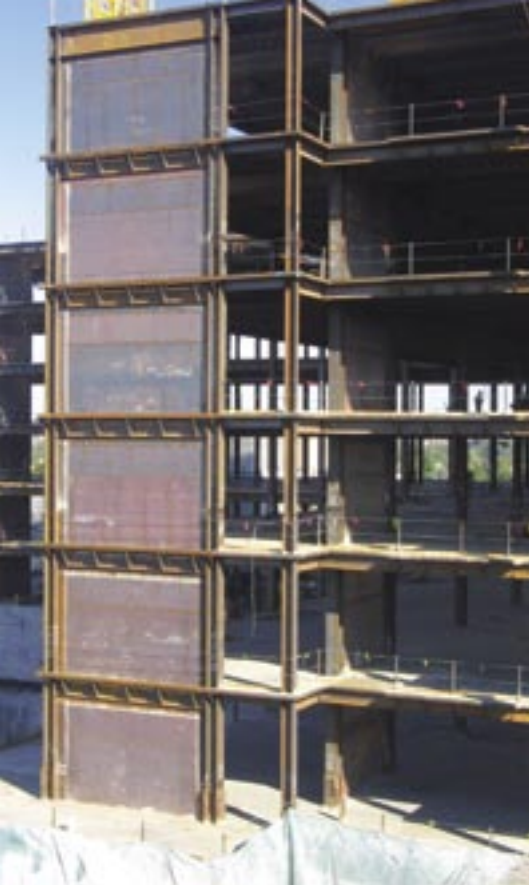
Shear walls are strategically located around the stair and elevator shafts and at solid exterior walls in order to avoid penetrations from doors and windows.
