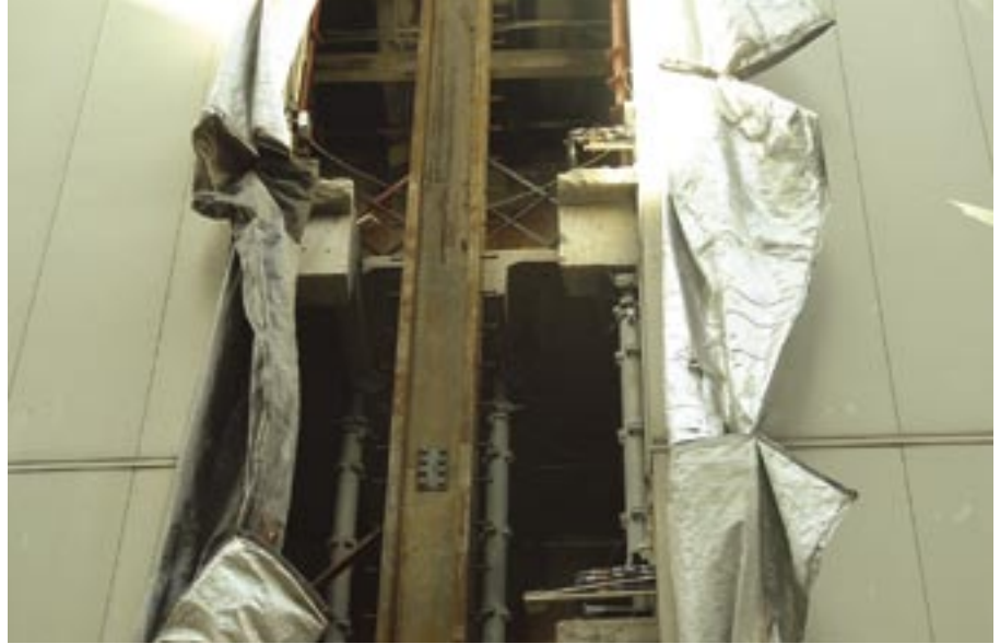
The existing concrete floor system and spandrel beams were shored and then saw-cut to make room for the composite columns. In the final configuration, the existing concrete framing is support by steel brackets and saddles welded to embedments cast into the composite column.
