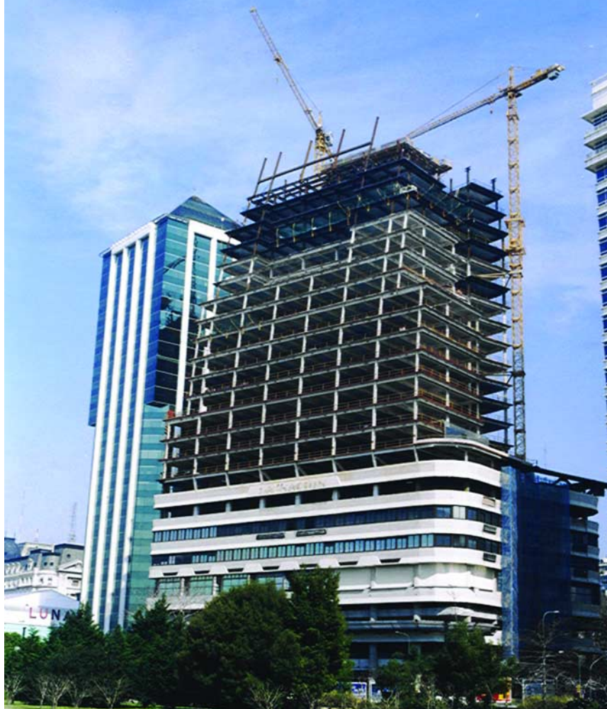
The structural steel members for columns, beams and girders are ASTM A572 Grade 50 steel. All connections are designed as bolted connections using high strength A-325 and A-490 bolts. The column and truss members at the transfer floor system are W14s.
